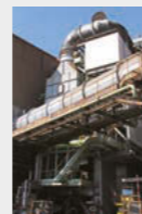
Exhaust heat recovery system
